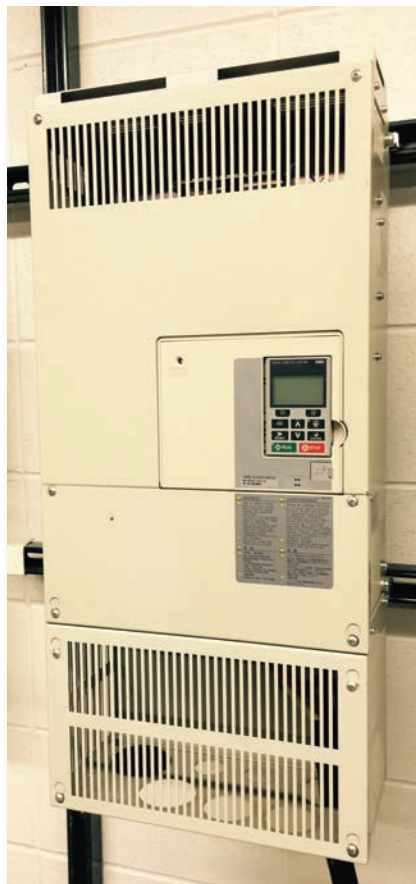
Figure 1: Users select variable frequency drives (VFDs) to control motor speed and reduce energy consumption. All graphics courtesy: Yaskawa America Inc.
